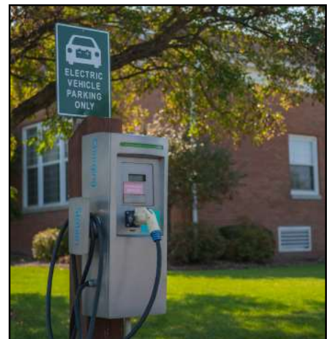
EV charging station at Penfield Town Hall campus. Penfield was the first municipality in Monroe County to install one on its property.
